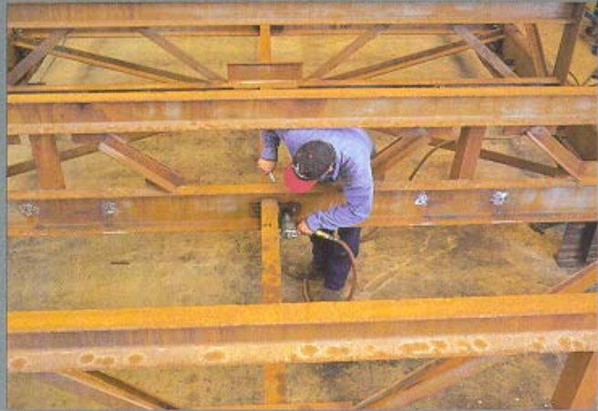
Upgrades are made to ensure the rebuilt traveling water screen will provide years of dependable service.
